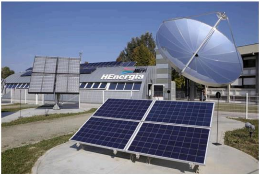
Figure XI.-PDC installed at HEnergia center for cooling [71].
